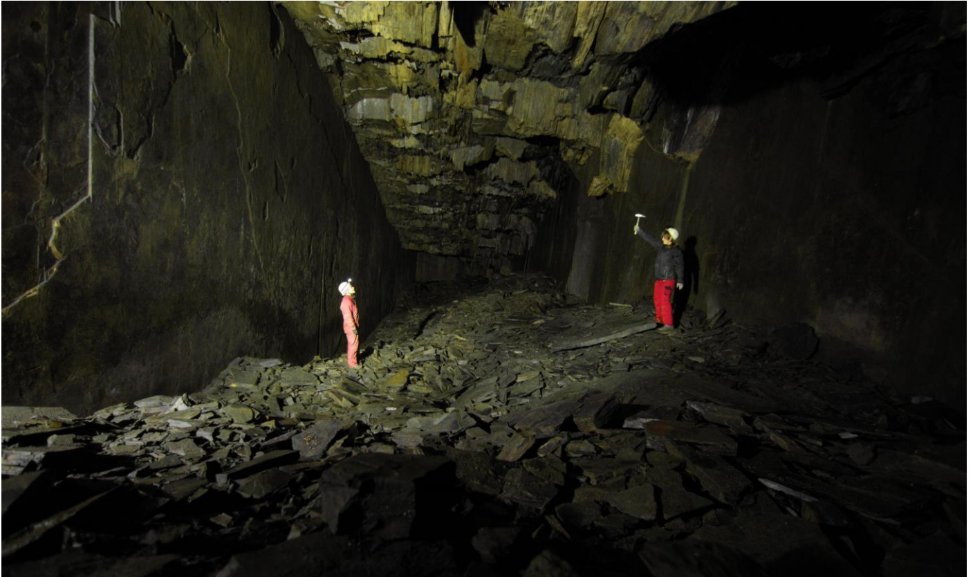
Figure 2: One of the large rooms after clayey slate extraction within the Woodboys mine in the Nížký Jeseník Upland. Photo: Jan Lenart, 2018
