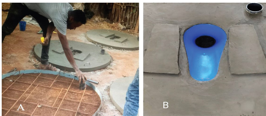
Figure 5: (a) Circular concrete slab and (b) rectangular concrete slab with plastic pan. (Source: Mamo & Novotny, 2024)
