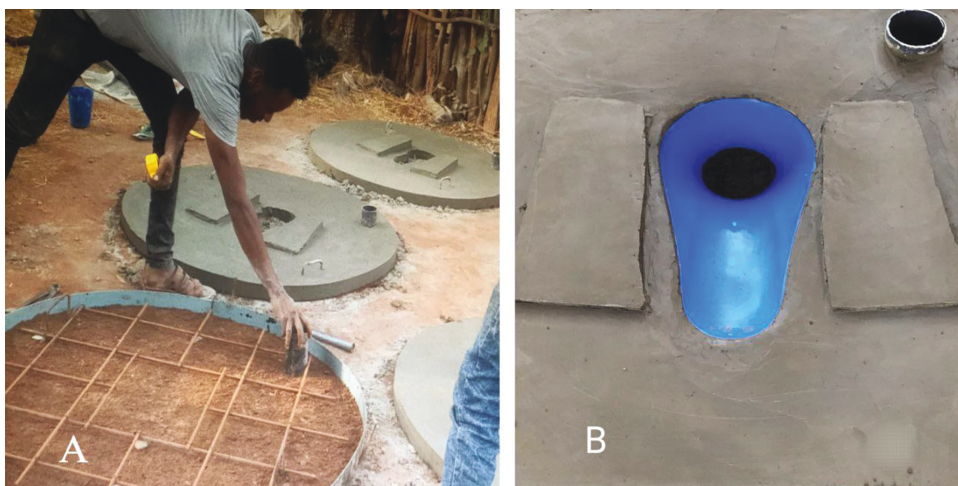
Fig. 1: (a) Circular concrete slab and (b) rectangular concrete slab with plastic pan.
