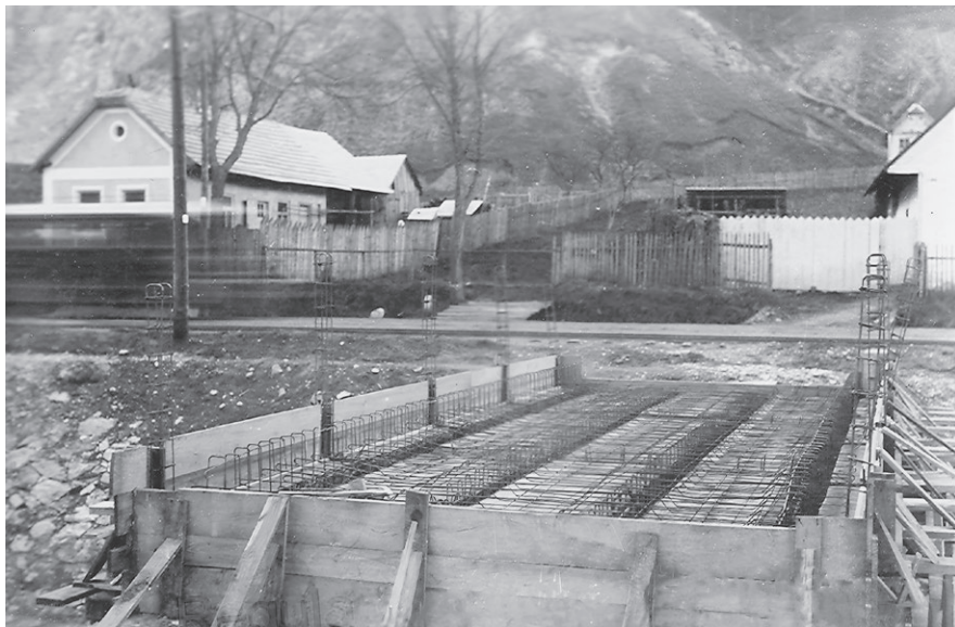
Fig. 4: The regulation of the Teplička stream in Trenčianska Teplá, 1930s. In the background on the right-hand side the gable of Štefan Stojka's house is visible.
